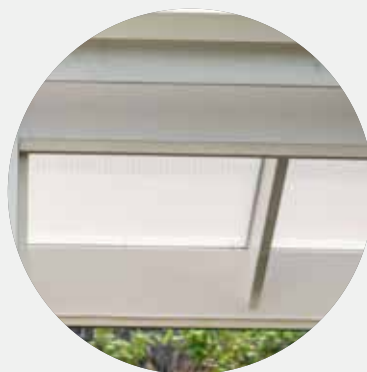
Lysinnslipp i taket
