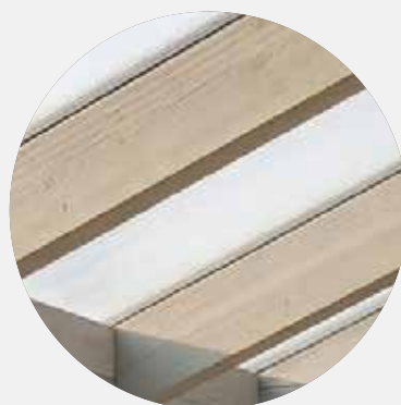
Lysinslipp i taket
