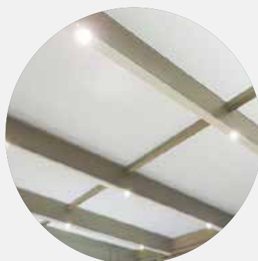
Lysinslipp i taket
